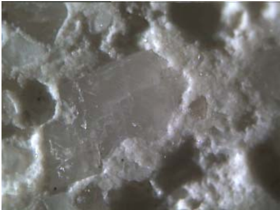
Figure 21 – Aggregate Exposure of Heavily Etched Plaster
