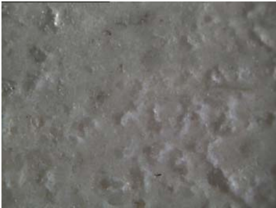
Figure 17 – Aggregate Exposure of Unetched Plaster (Unexposed to Water)
