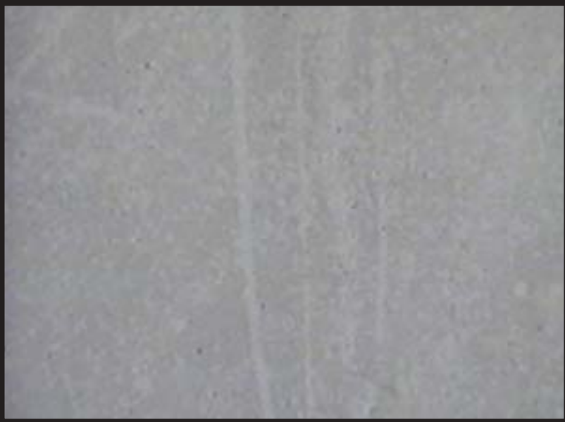
oB-00005Do – Drip lines on wall
