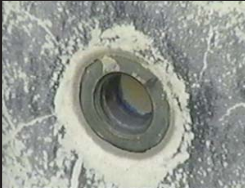
oB-00005Dn – Discoloration around fitting
