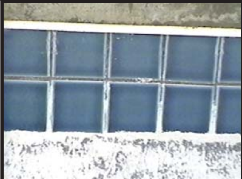
oB-00005Db – Sloppy cleanup – whitened plaster over grout below water level
