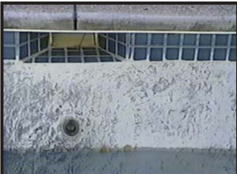
oB-00005Da – Sloppy cleanup – whitened plaster over grout below water level plus discolored wall
